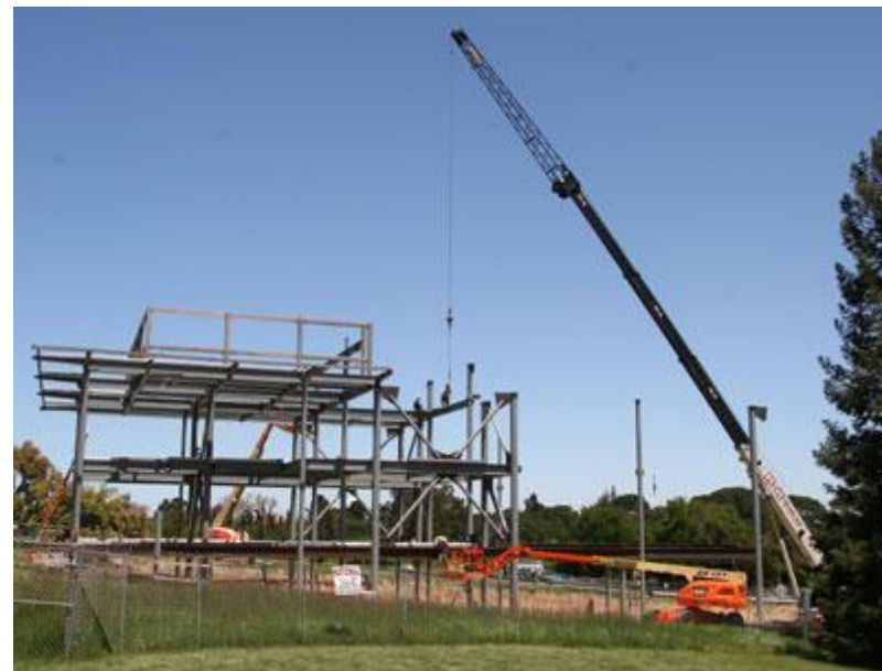
The Kavli Institute is quickly rising to its full three story height. Construction should be completed by early 2006.
