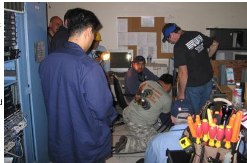
SLAC electricians convert 480v from diesel generator to 120/208v to be used for power in Building 50 to bring network and servers back temporarily. Shown left to right: Brandon Mai, Fikrit Alisic, Francisco Castillo, Ricardo Delgado, George Quilon and Richard Altieri.
