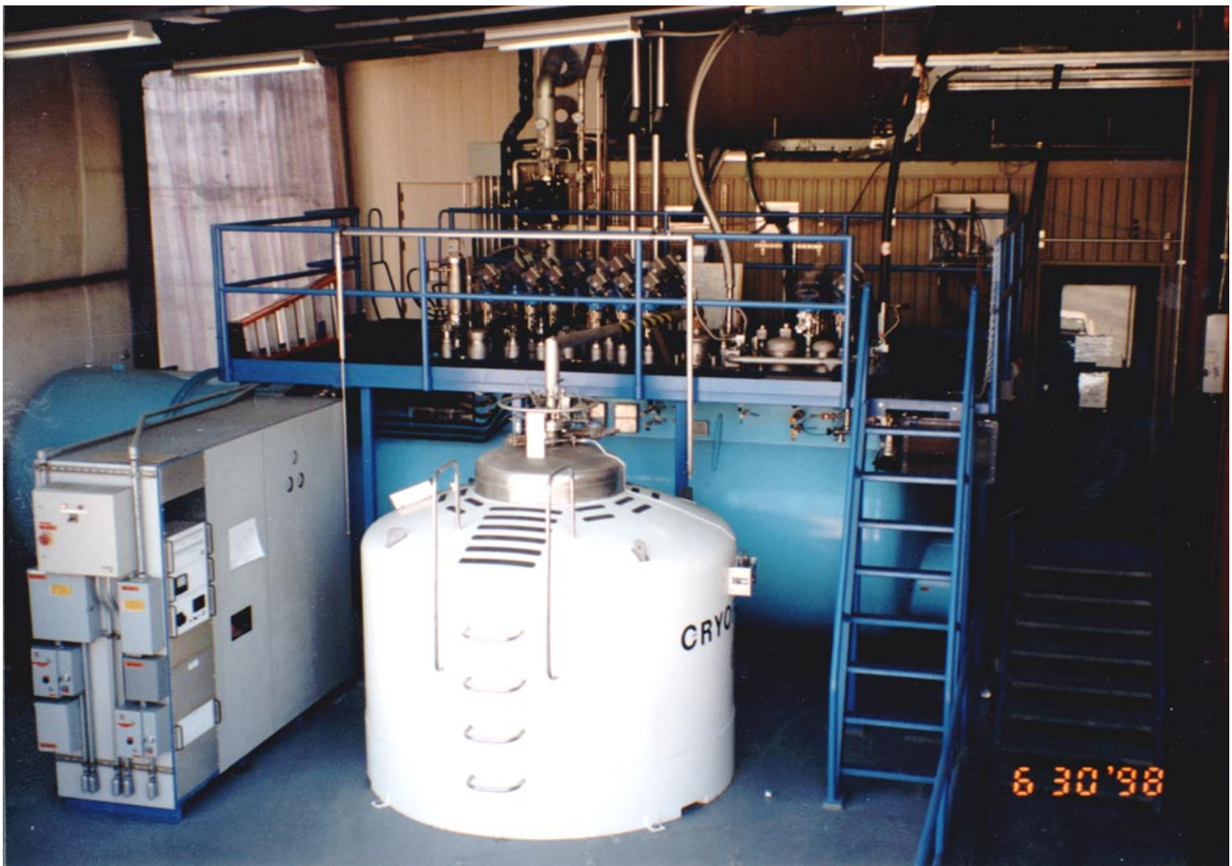
Figure 6 The completed cold box installed at SLAC.
