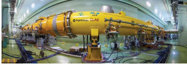
Figure 2: S1-Global cryomodule installed in the underground STF tunnel at KEK.
