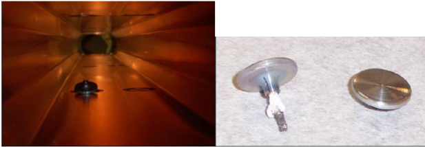
Figure 19: A button of an upper BPM fell off onto a lower button (left plot). Melted feed-through of a lower button and the fallen upper button (right plot).
