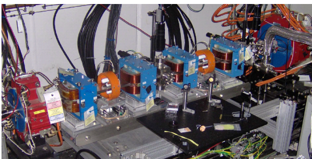
Figure 4: Image of C2 after installation.
