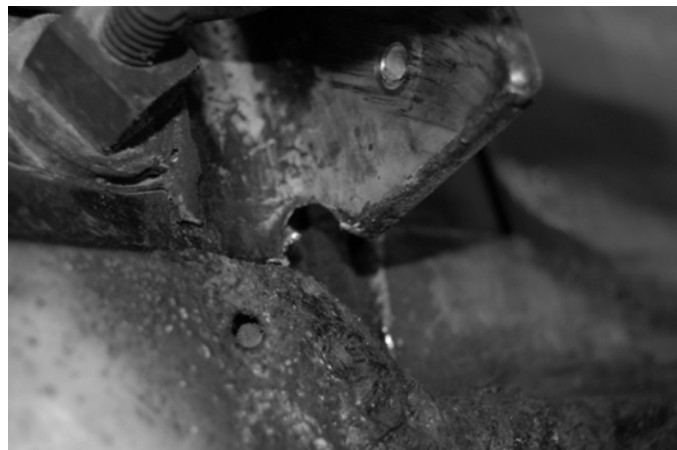
Figure 4. Photograph of a flat-pack switch plate failure at SNS due to arcing between two close conductors.
