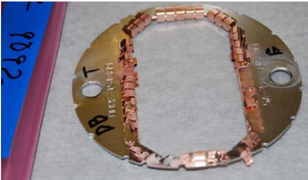
Figure 8: Melted omega seal of the 9092-flange.
