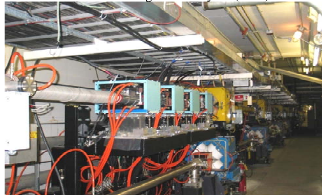
Figure 1. Detail of the newly installed 4-dipole chicane in the PEP-II LER in IR12 (upper beam line). The clearing solenoid can also be seen upstream of the first magnet (left side of the picture).
