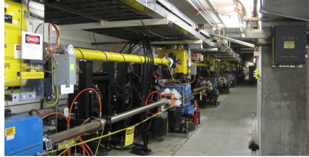
Figure 3. LER vacuum chamber in IR12 (upper beam pipe). The outer clearing solenoid can be seen.
