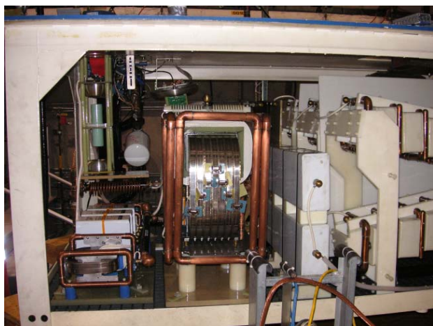
Figure 2: View of doubler capacitors and output filter choke
