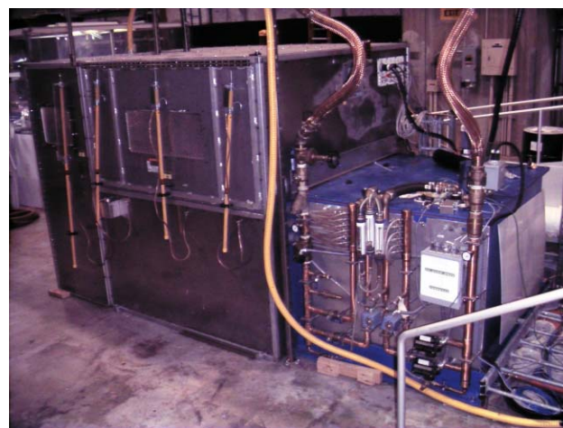
Figure 4: 15 MW output converter-modulator
