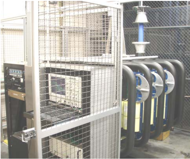
Figure 1: Photo of the SLAC Marx Modulator with 10 of the 18 cards installed.
