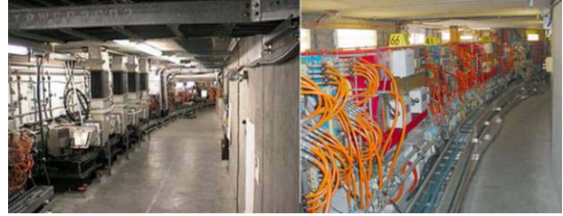
Figure 1: The rf straight section (left) and north arc (right) of the SPEAR 3 tunnel.
