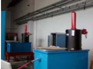
Figure 2: SPARC klystrons with oil tanks installed in the SPARC building (upper facility room or klystron hall).
