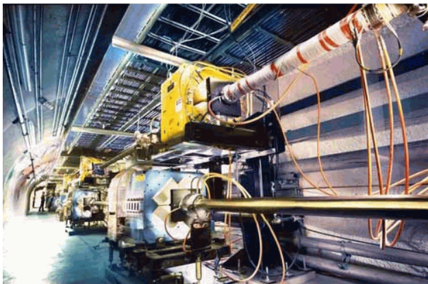
Figure 1 View of the PEP-II tunnel.
