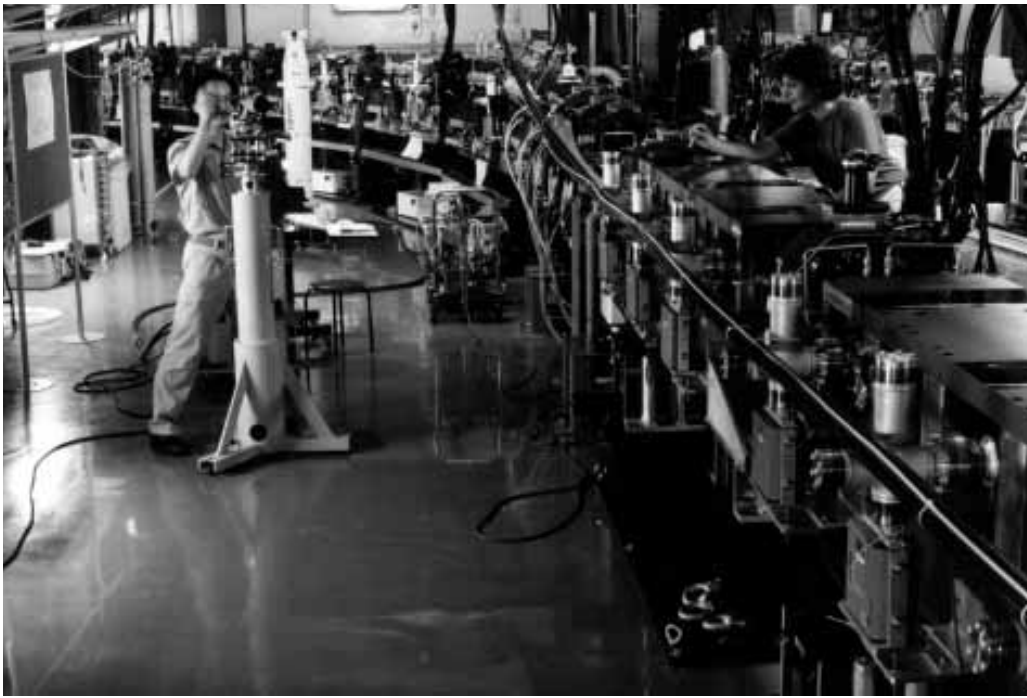
A portion of the Accelerator Test Facility Damping Ring. High precision alignment of individual components is important, although an automatic beam-based alignment system will ultimately be used.
