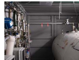
HFE-7000 storage dewar and transfer lines
