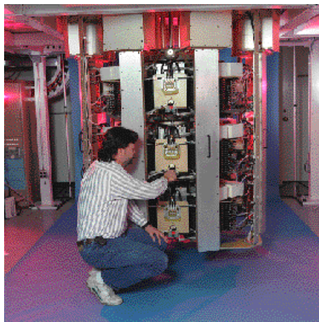
Fig. 5. The three-stage ARM modulator assembly which produces 45 kV (open circuit) at 4.8 kA and 1 MHz repetition rate.
