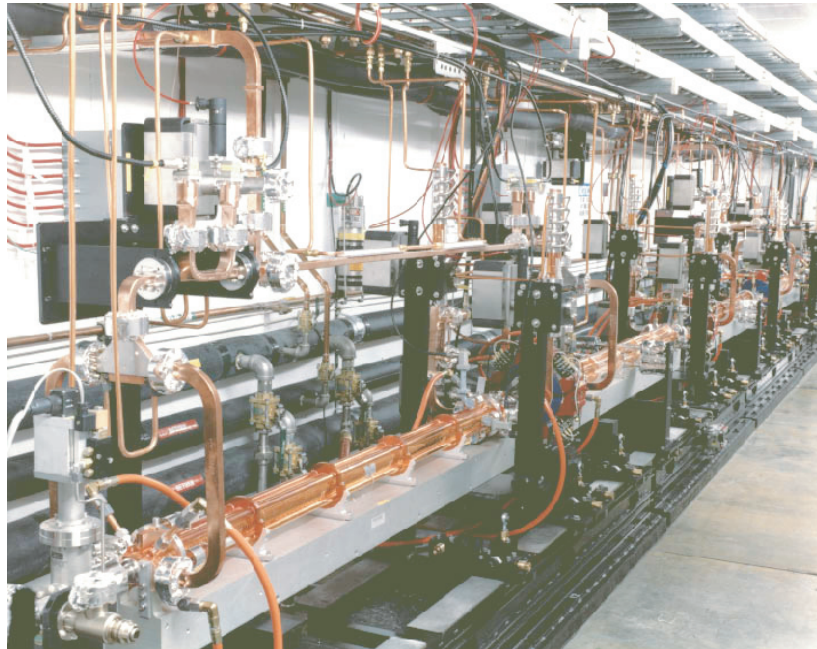
FIGURE 5.8. Photograph of the beam line in the NLC Test Accelerator.
