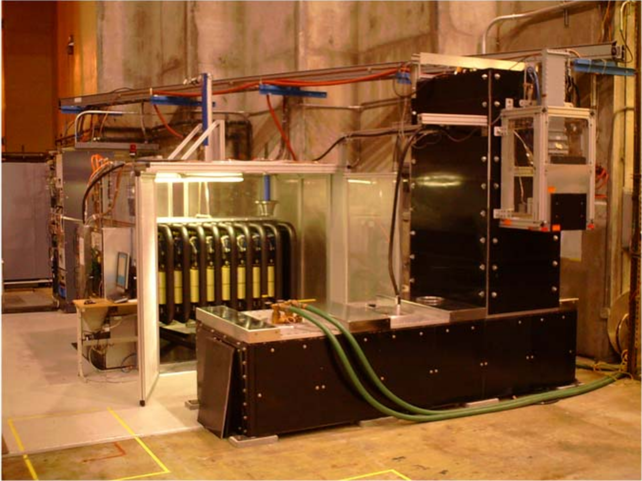
Figure 3. L-band test station; 10 MW klystron (right), Marx modulator (center), Rf controls (left).
