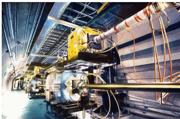
Figure 1 View of the PEP-II tunnel.
