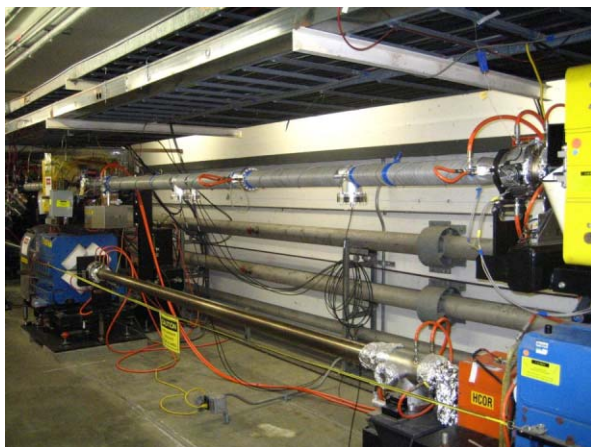
Figure 2: Detail of the LER vacuum chamber in IR12 (upper beam pipe). The inner clearing solenoid can be seen.
