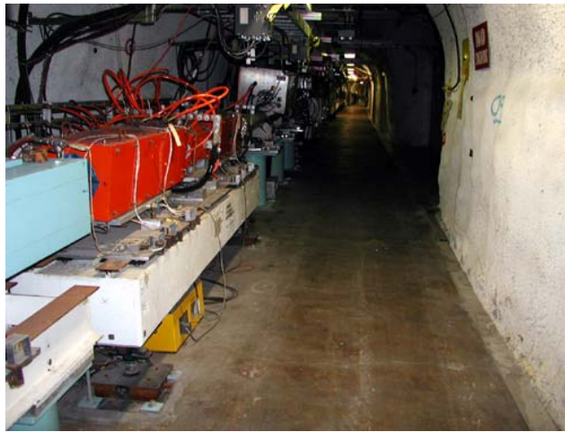
Fig. 1 - SLC Accelerator Tunnel and Magnets to Test Laser Scanner
