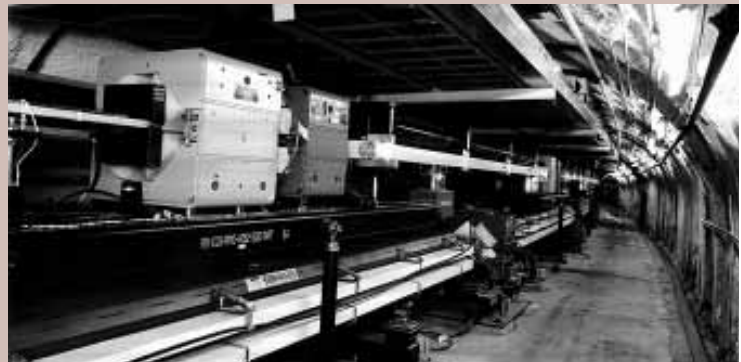
A view down the tunnel of the PEP-II B Factory. The positron ring sits just above the electron ring.
