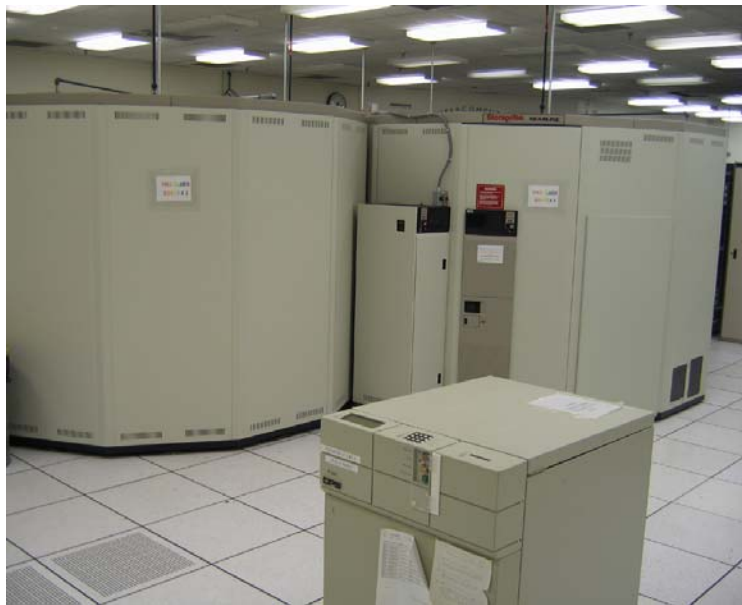
Figure 2: BNL HPSS Mass Storage System
