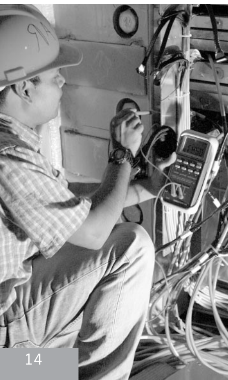
SLAC Research Associate Tests New Muon Detector Planes Being Installed in August 2004.
