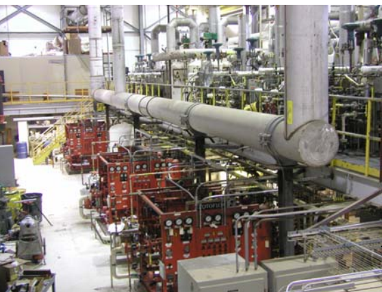
Turbines (Refrigeration Production)
