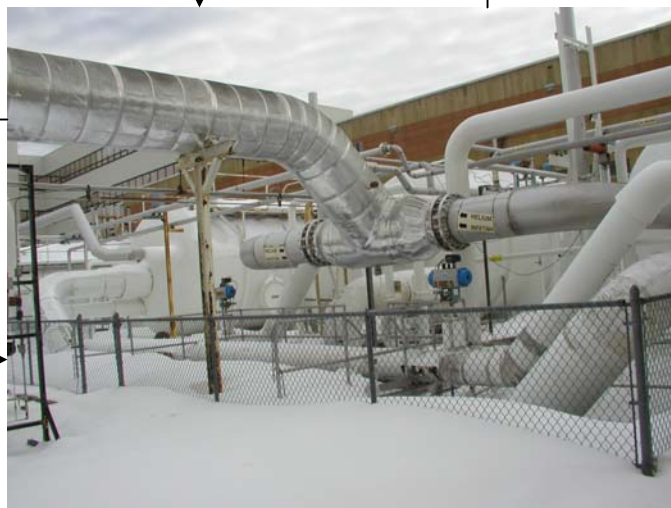
Cold Boxes (Heat Exchangers – Energy Exchange)
